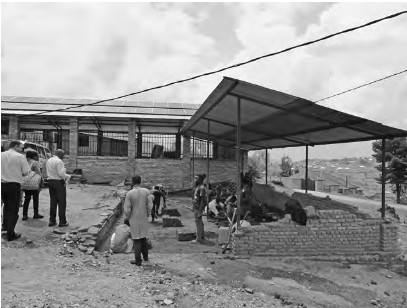
Ruanda: Solar-PV-Stromanlage in Shougwe
